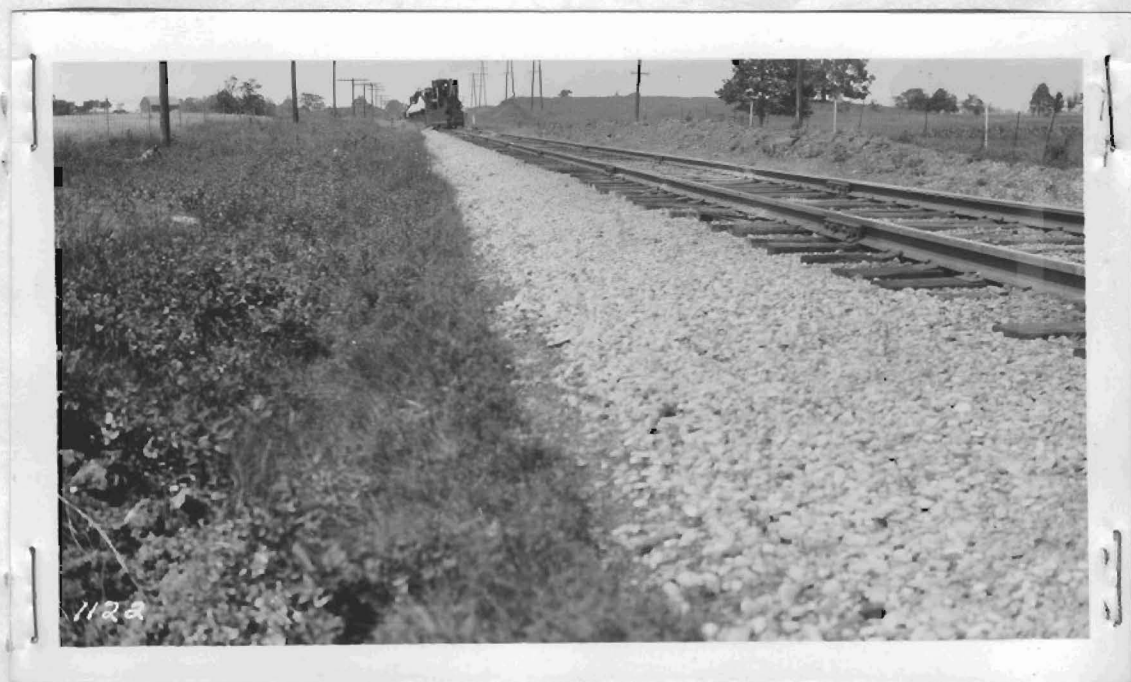
A view of the Type A Spreader-Ditcher before starting the ditching operation.
