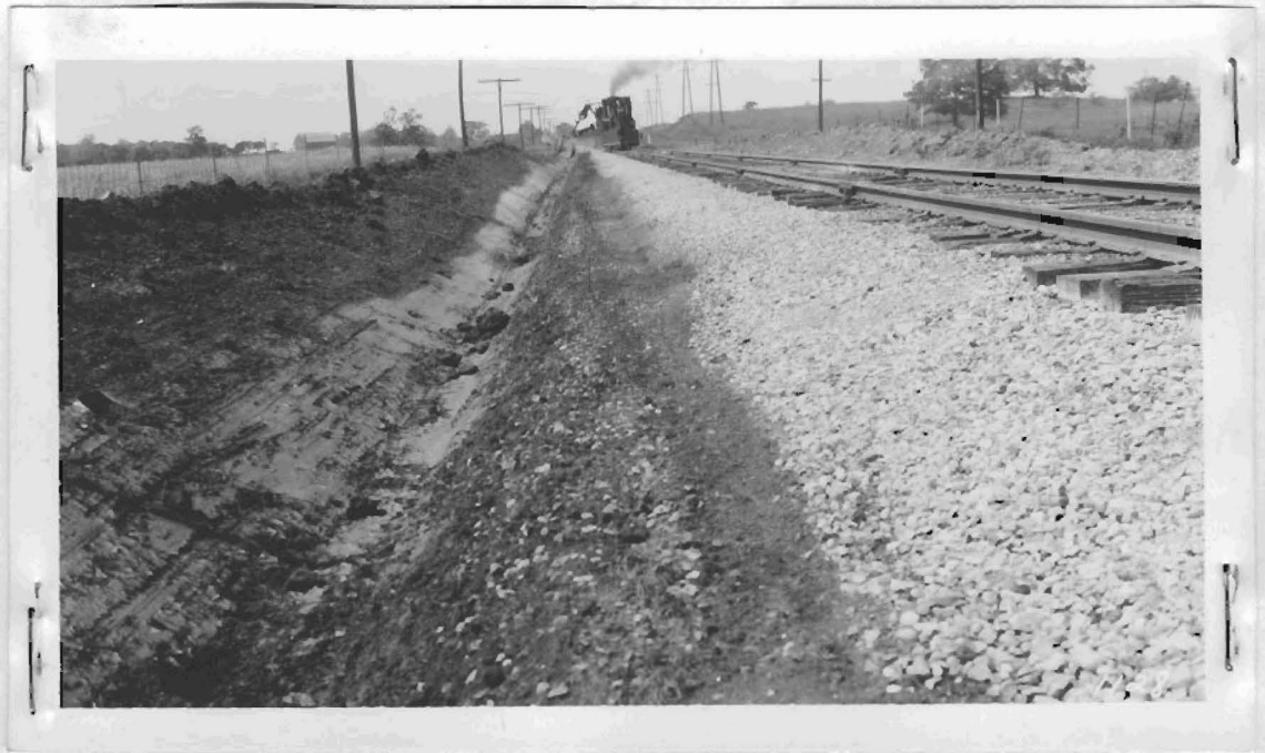
This picture taken after the JORDAN has passed through the cut a couple of times. This cut necessitates another trip through in order to complete the work.
