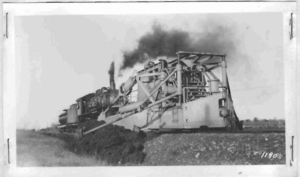
Another view of the same operation showing the dirt being carried out on the fill. In operating a Type A JORDAN in carry wing form, we widen the cut and widen the fill in the same operation. The cost of handling dirt in this form is at a minimum.
