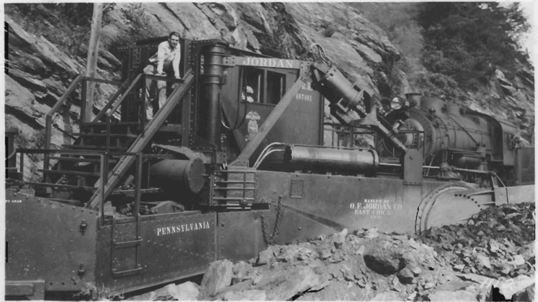
Side view of a Type A JORDAN Spreader-Ditcher machine converted in spreading form showing left wing leveling material adjacent to the track preparatory to laying the second main line.
