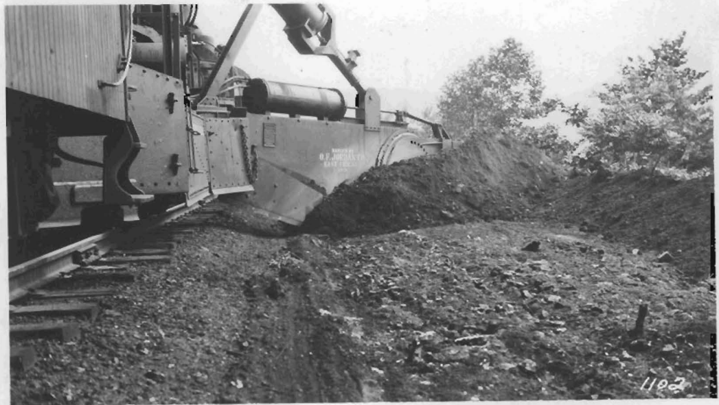
Another view of the same operation as above showing the operation taking form. The Type A Spreader-Ditcher is also used in this particular job for spreading fills thereby shaping the ballast and leveling the sub-grade.
