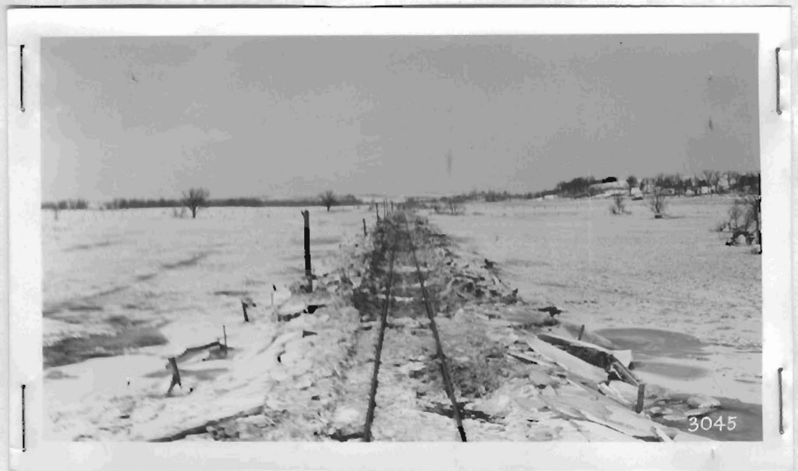
This view shows another section of the track which was opened by the Type A. The main wings were not opened to spread the ice further away from the track due to the fact that the ice being plowed in this manner would break telegraph poles and fence poles.
