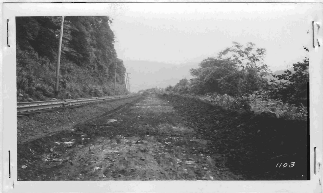
A view of the finished operation. Later ballast was dumped from side dump cars, leveled again with a JORDAN Spreader making the roadbed ready for the application of ties and rails.
