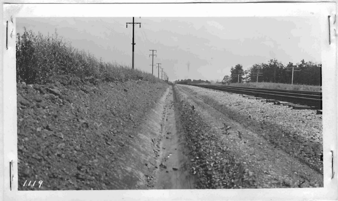
This view illustrates the neat work which can be accomplished with a Type A JORDAN Spreader. Your attention is called that all cuts ditched out in this way give you perfect drainage also during the winter months aids materially in handling snow.
