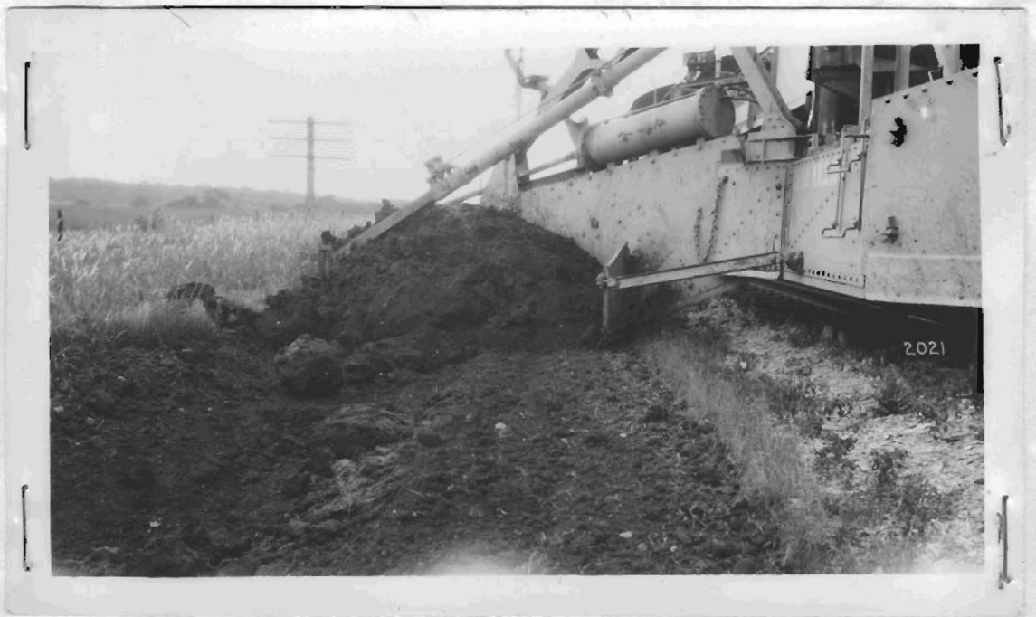
A Close-up view of a Type A JORDAN showing the right wing converted into carry wing form. Note the dirt carrying capacity and also the small ballast carry wing which prevents the dirt from coming up on the ballast.
