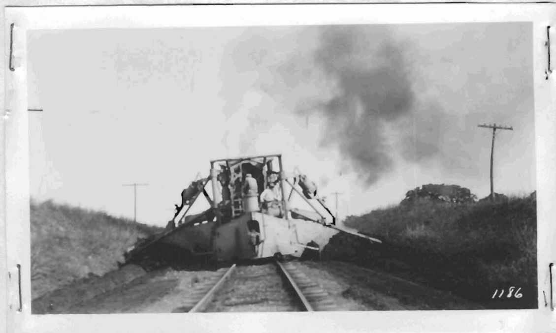
This view shows a Type A JORDAN converted in carry wing form. The machine is used in this form in dragging dirt out of a cut. Both wings can be used on single track operation.
